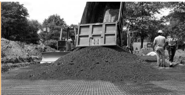
Figure 9a: Dumping aggregate fill on top of BX Geogrid over soft subgrade.
