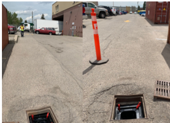
Figure 2 shows the loading dock as well as the visitor and employee parking area near the catch pit
