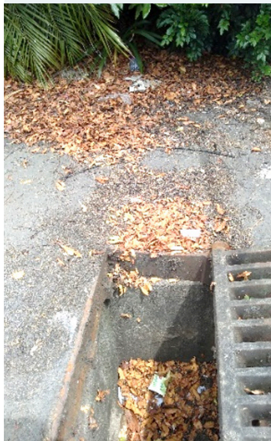
Figure 7 Litter within leaves around a catch pit prior to the quick and easy installation of a LittaTrap™.
