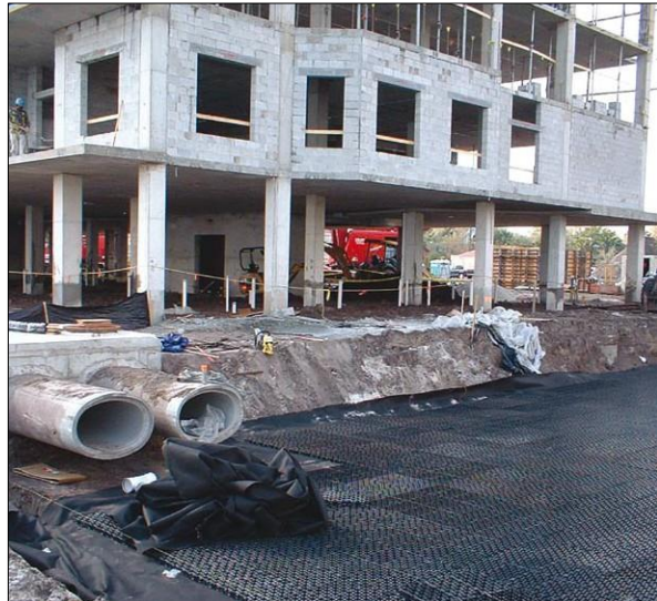
Inlet pipes for Atlantis® detention tank.
