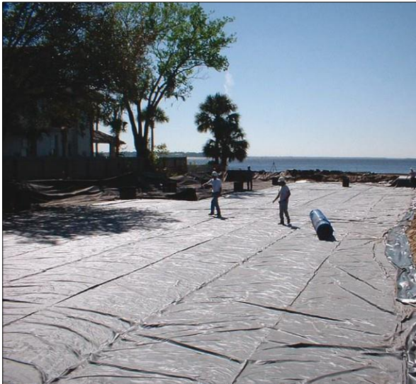
52mm Atlantis® Drainage Cells covered with geotextile in preparation for Atlantis® Matrix® Tank Modules.
