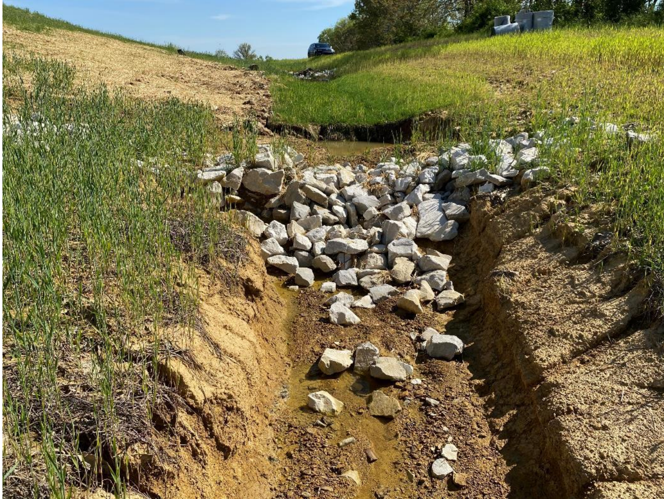
May 1, downstream rock check dam damage
