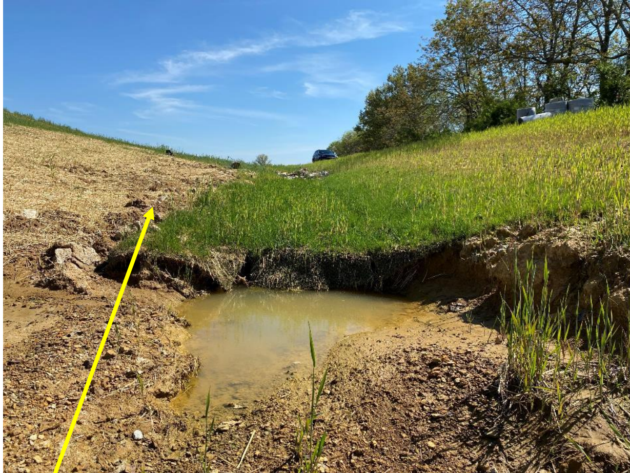
May 1, note in-filled gully left side of test section
