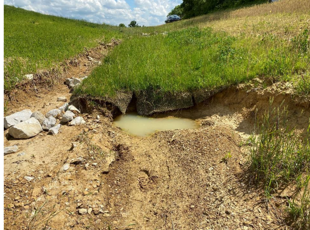
May 28, in-filled soil washed out, rock deposited from check dam upstream
