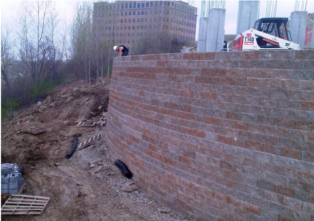
The random placement of three different colored Mesa Units gave the finished wall a unique appearance.
