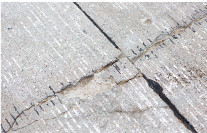
PROBLEM Excess cracking on High Street in the City of Freeport needed to be addressed and fixed
