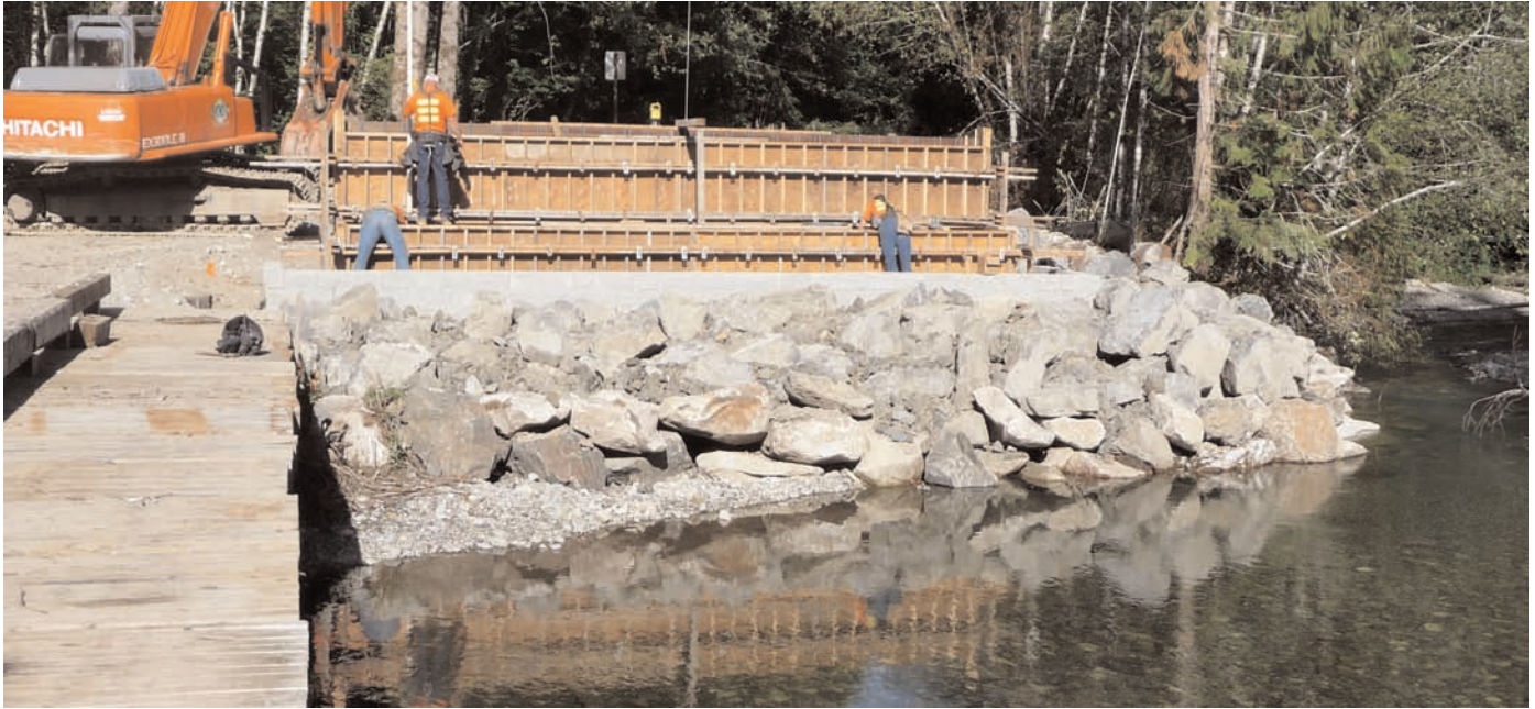
Finished bridge abutment constructed using a wrapped face and block wall with Mirafi® HP570.
