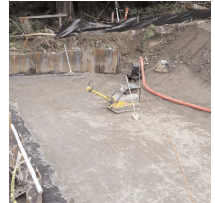
Construction of the new MSE bridge abutment using Mirafi® HP570 and thin lifts of compacted fill.
