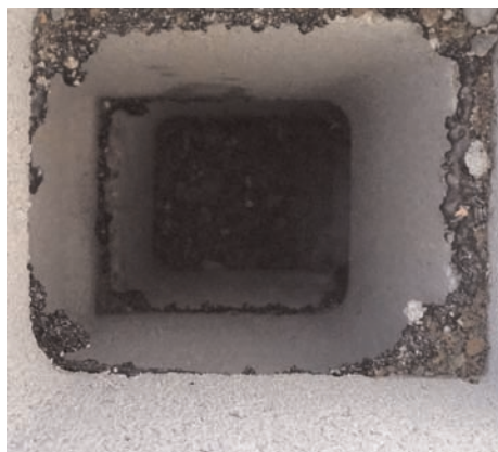
Blow torched, cut out center of CMU blocks where Mirafi® HP570 had been placed, to be filled with crushed rock.
