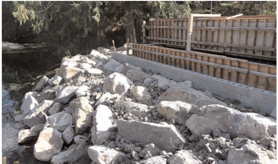
Finished bridge abutment constructed using a wrapped face and block wall with Mirafi® HP570.
