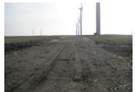
Road construction looking west using Mirafi® HP570 and 8" to 10" of limestone after 5 years.
