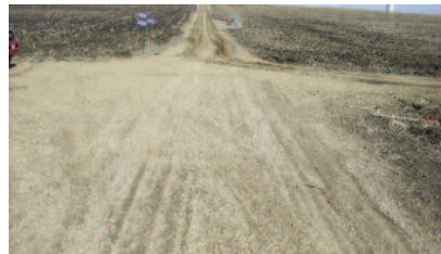
Road where soil cement and geotextile were used. Construction was completed and reviewed after 6 months. Note stone loss and rutting.
