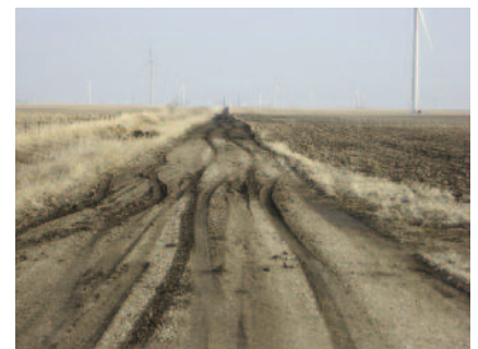
Road construction looking north using soil cement and 4" of limestone after 5 years.
