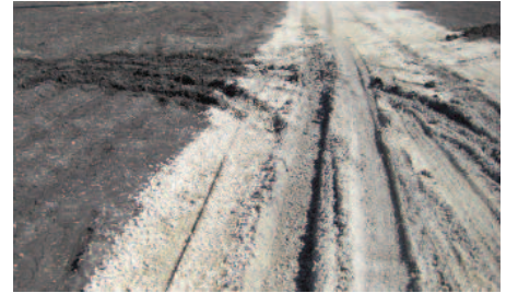
Break down of soil cement after 6 months due to freeze-thaw cycle and moisture.
