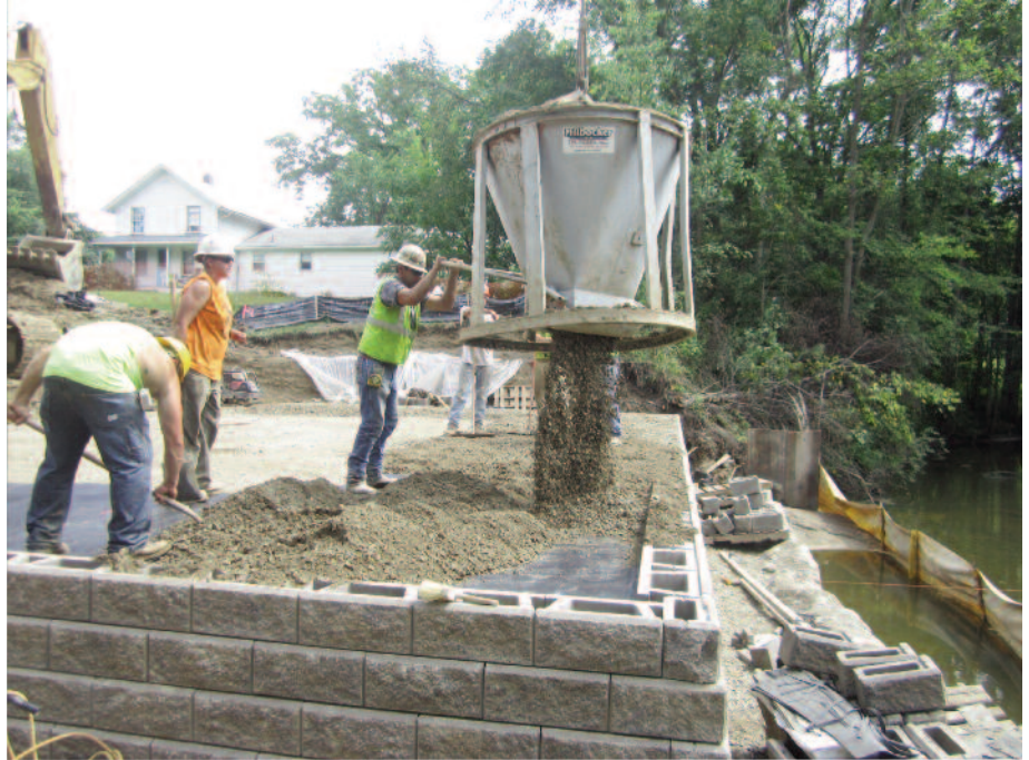
Stone is placed behind the block, on top of Mirafi® HP570. Care must be taken with loading until compaction is adequate.
