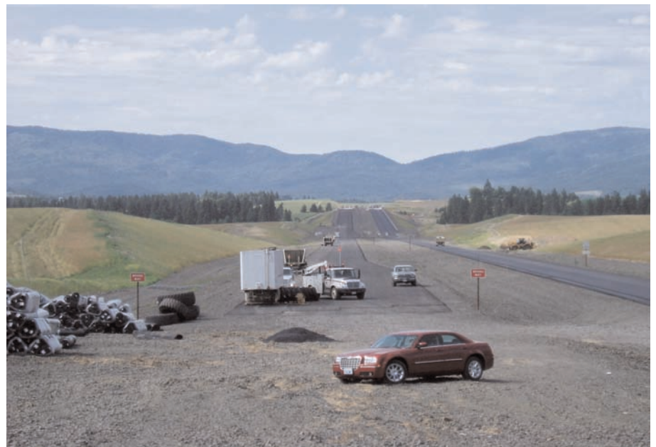
Picture of the newly completed roadway subgrade, just south of Worley, ID.
